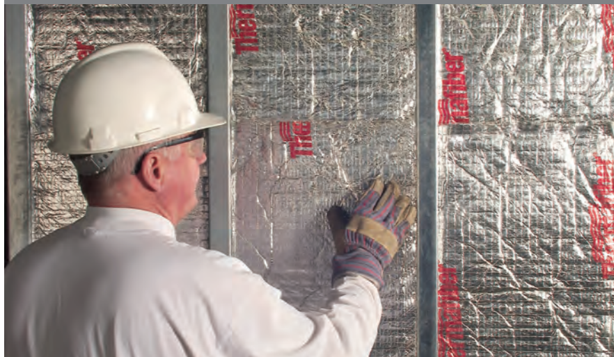
FS-25 with a vapor retarding foil facing is installed in an exterior stud wall.
